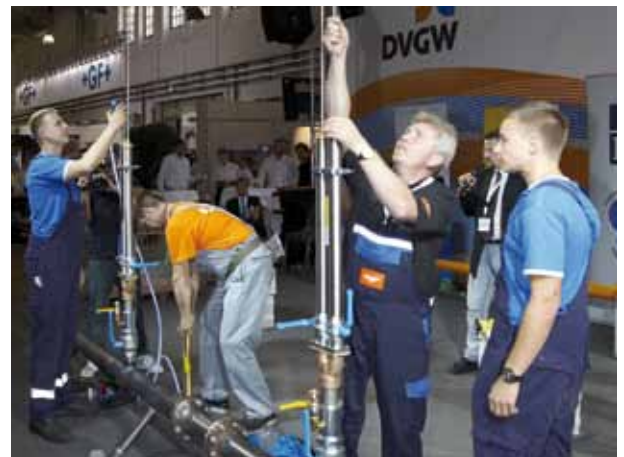
● Team spirit was called for in pipe tapping for the installation of a tee on a "hot" pipeline.
